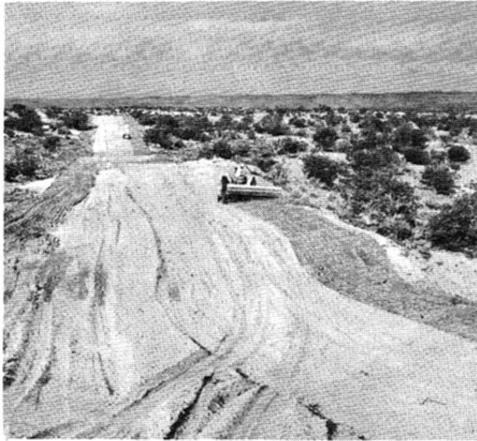
Reseeding of a pipeline lateral to crested wheat was one of the projects undertaken on the Huerfano Range Conservation Area. This is pinon-juniper type range, characteristic of millions of Western areas.
